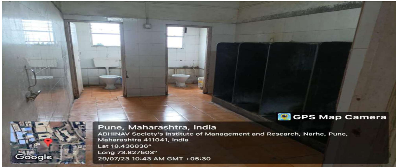
Water provision in the premises
