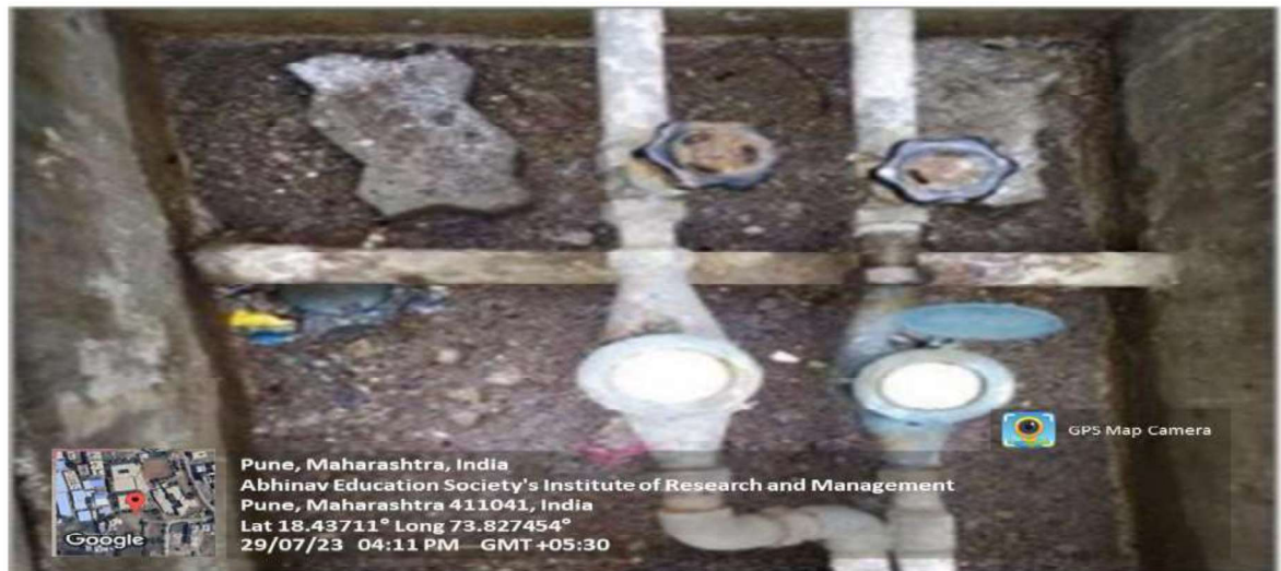
Water tank provision and connection meter in the premises
